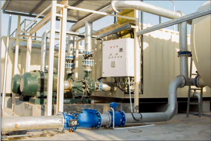
Figure 7.5. USAID-funded water treatment plant
